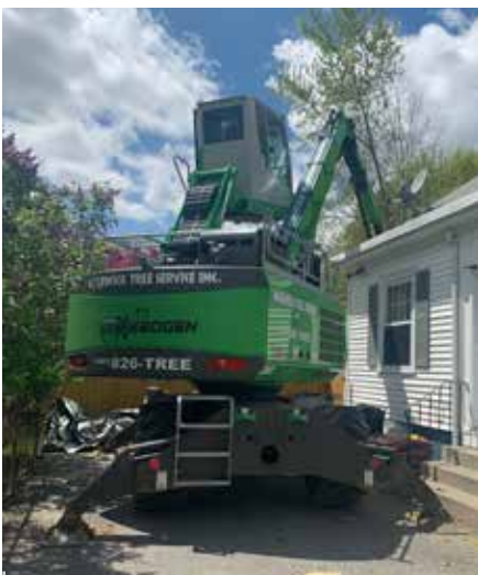
People came to watch Kyle working. With its reach and elevating cab, Kyle can “see” over the house.
