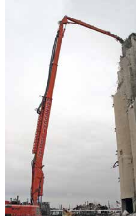
Equipped with a 182' (55 m) long reach boom & stick, the SENNEBOGEN 870 R-HD makes quick work of the site.
